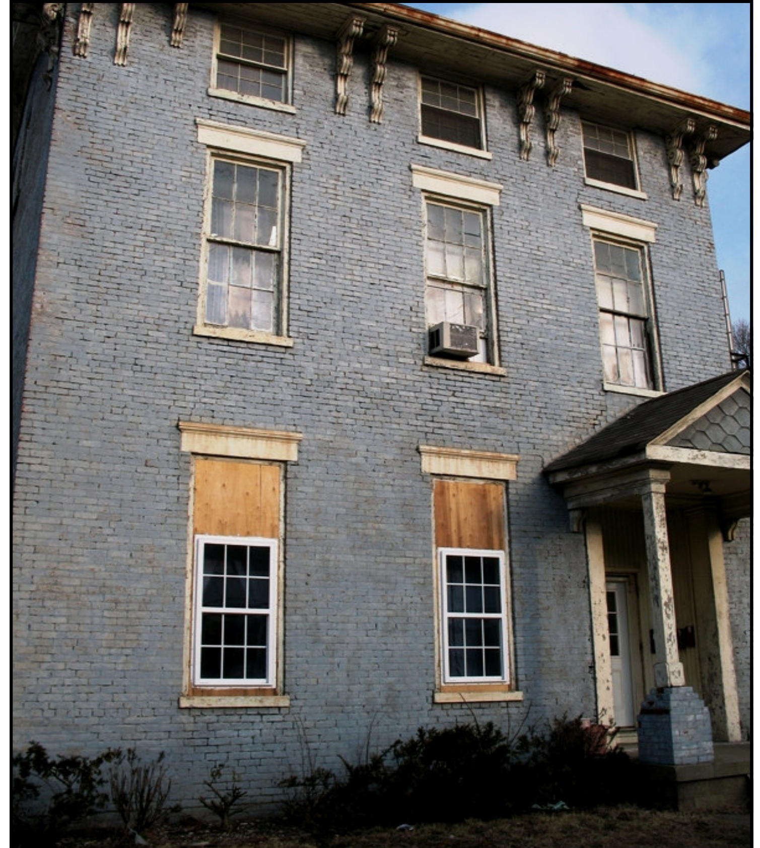
19th century Italianate style house Replacement windows do not match size, type or material
