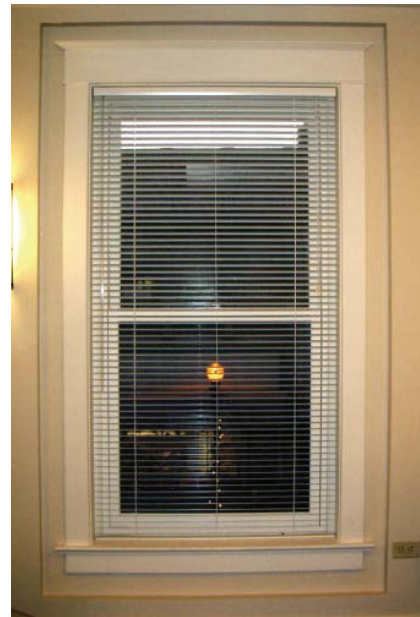
Fig. 20. The walls have been furred out inappropriately around the historic window trim creating an appearance the interior never had historically.
