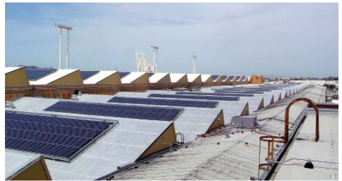
Fig. 23. Solar collectors installed in a compatible manner on low sloping sawtooth monitors. Top Photo: Neil Mishalov, Berkeley, CA.
