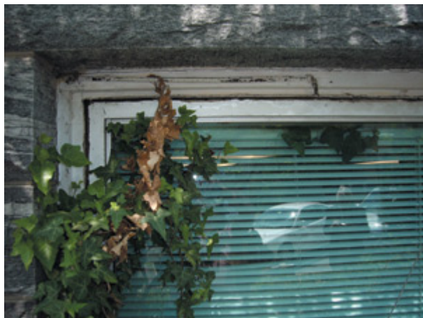
Replacing sash while ignoring the primary sources of infiltration can have detrimental and costly results.
